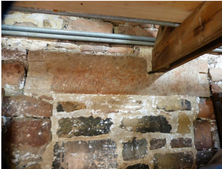
Plate 5: Blocked doorway [5] in the external south face of the barn (now within lean to). Note the reddened burnt stone of the jambs and lintel and above
