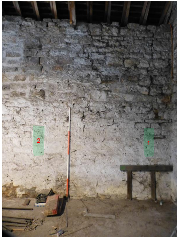
Plate 1: Inner face of south wall of barn; west end. Feature toned in green and numbered as per catalogue
